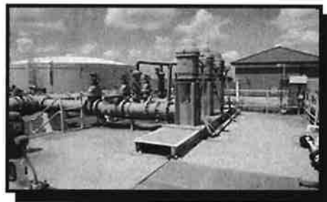
Carrousel System - Transfer Pump Station
