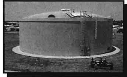
Reclaimed Water Ground Storage Tank
