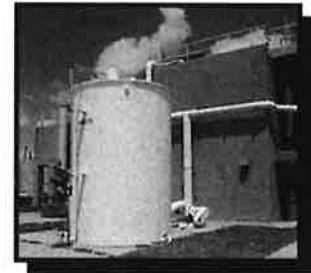
Pretreatment Structure Odor Control System
