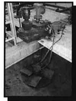
Grit Removal System
