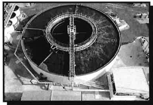
Ring-Steel Biological Treatment Unit
