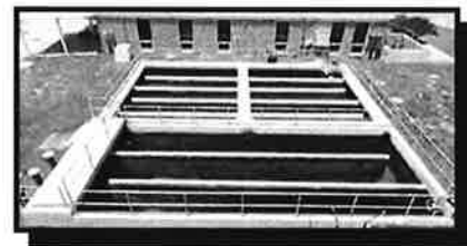
Chlorine Contact Chambers (CCCs)
