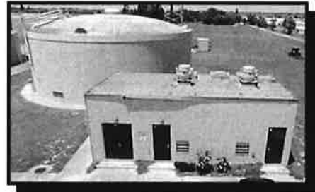
Reclaimed (Reuse) Water Pump Station
