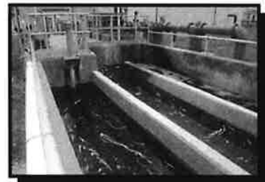
Chlorine Contact Chamber (CCC)
