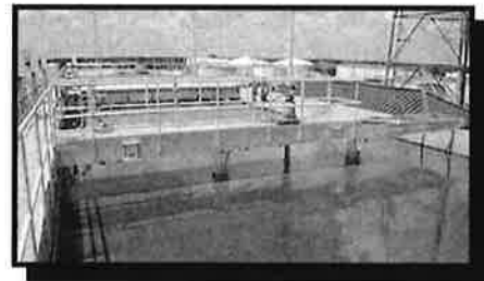
IFAS BNR System: Primary Anoxic Basins
