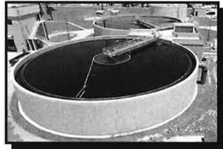
Secondary Clarifiers - Ox. Ditch System
