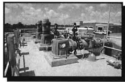
IFAS System - Transfer Pump Station
