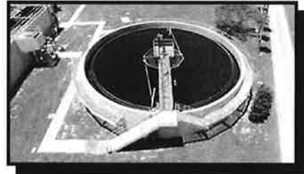
Secondary Clarifier - Conv. ASP System
