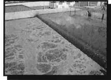
Aerobic IFAS Basin
