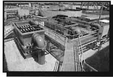
Tertiary (Disc) Filters - IFAS System
