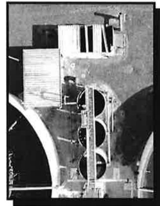
Tertiary Filtration System
