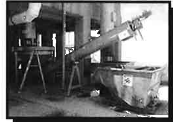
Grit Washing/Dewatering Unit
