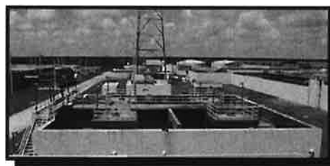
Carrousel BNR Treatment System: Anaerobic Basins
