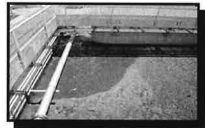
IFAS Secondary Anoxic Basin
