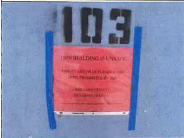
County Sign Indicating Building is Unsafe
