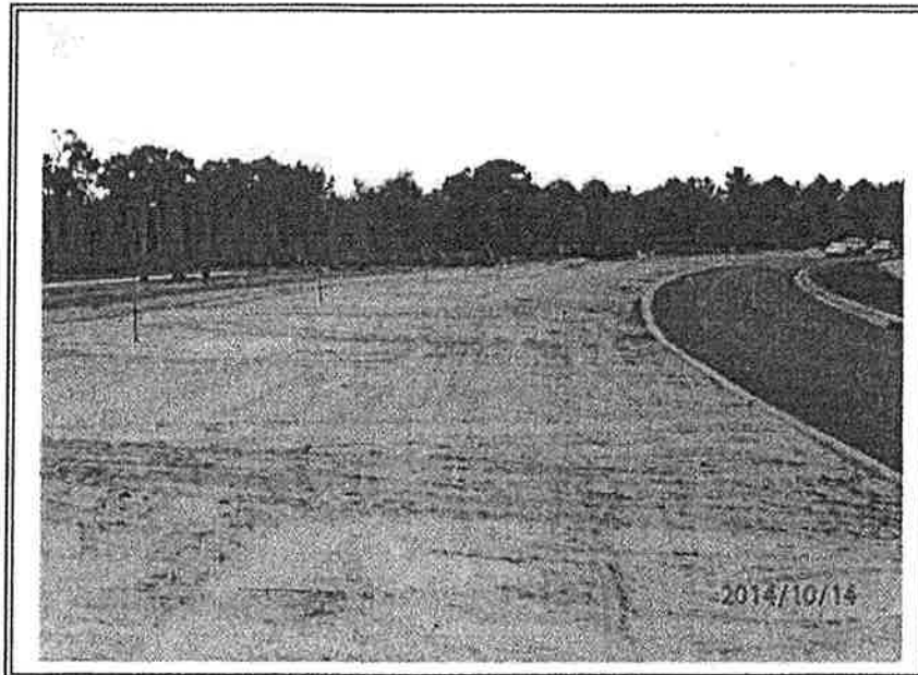
Lake Andrew Drive Phase 2A unfinished median
