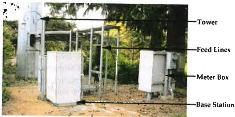
Figure 1: Example of 1900 MHz Wireless Infrastructure Ground Equipment
