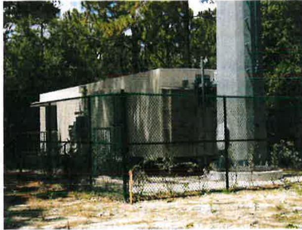
Figure 2: Example of 800MHz Wireless infrastructure Ground Equipment
