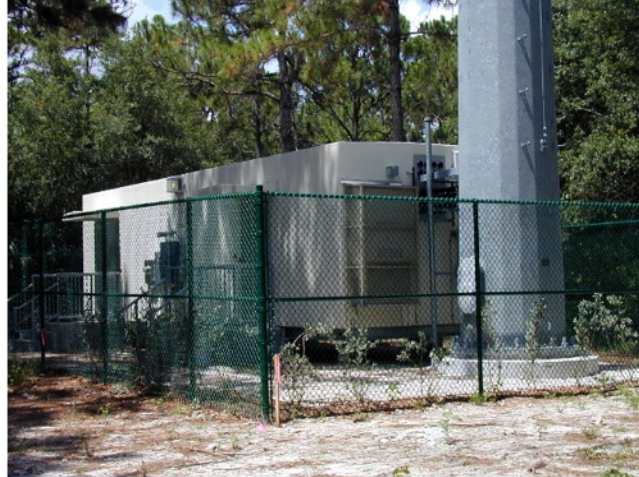
Figure 2: Example of 800MHz Wireless infrastructure Ground Equipment
