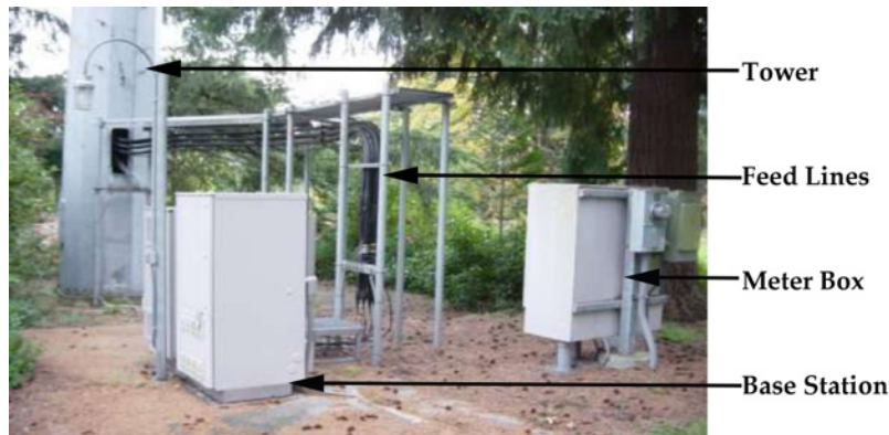
Figure 1: Example of 1900 MHz Wireless Infrastructure Ground Equipment
