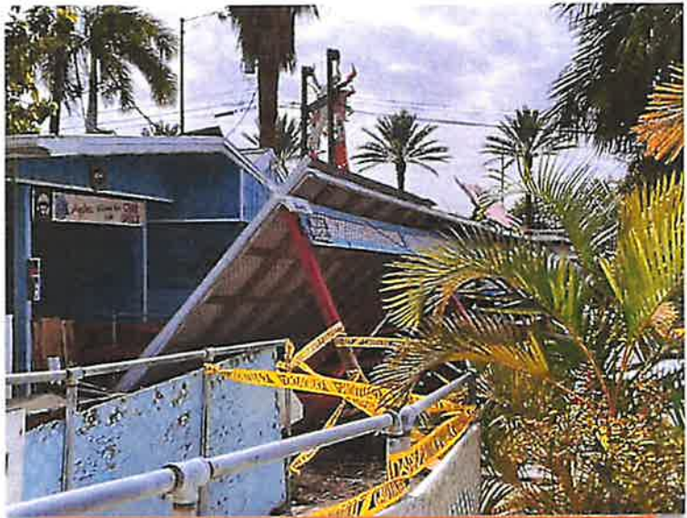
Ms. Apples Crab Shack at Blue Crab Cove/Griffis Landing sustained significant damage from Hurricanes Helene & Milton in 2024
