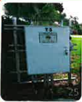
Lift Station Control Panel Modernization
