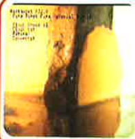
Collection system inflow and infiltration (I&I), leaking and causing higher flows
