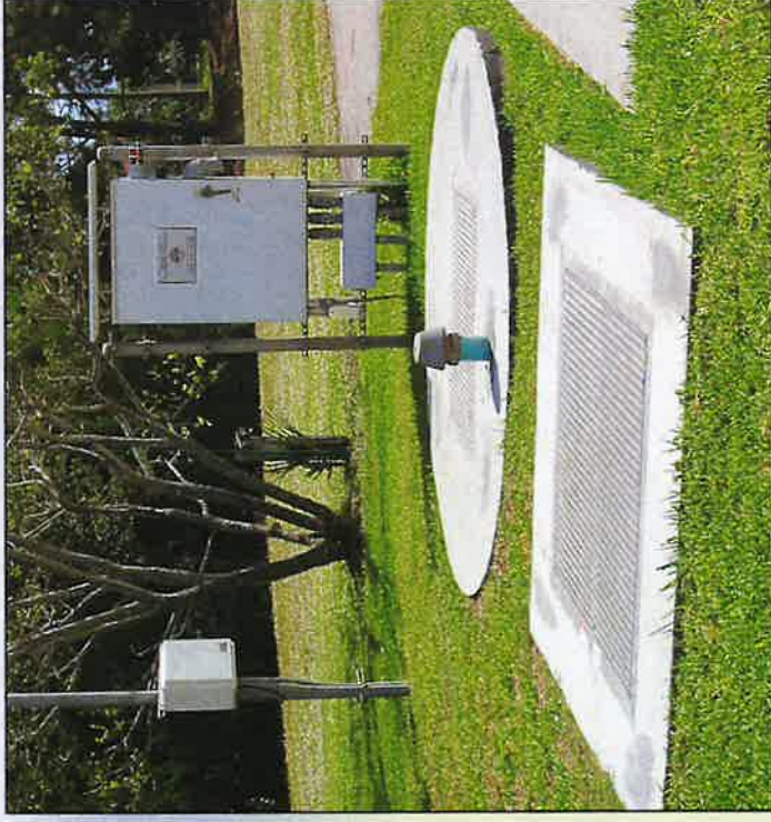
Figure 4 – Typical BCUCSD Lift Station
