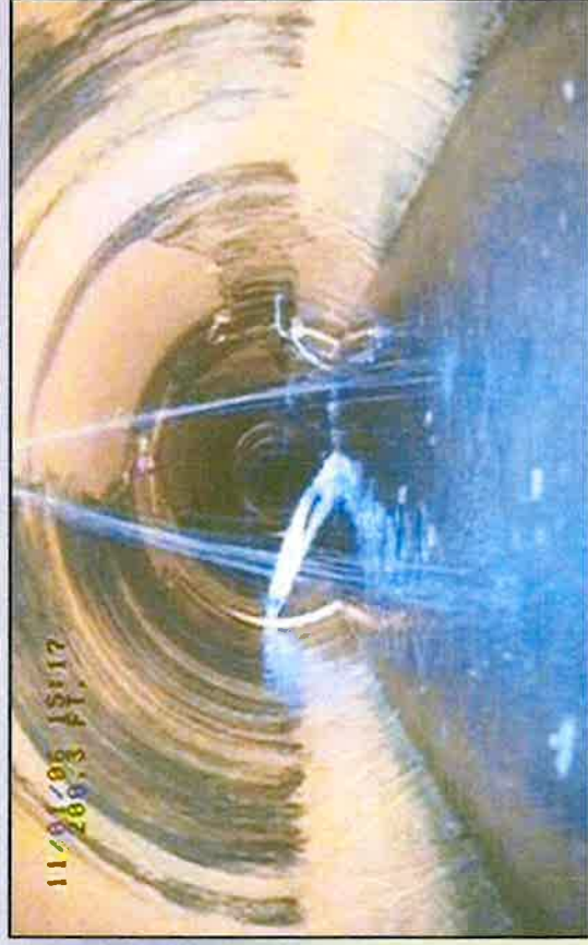
Figure 16 - Groundwater infiltration in sewer pipe
