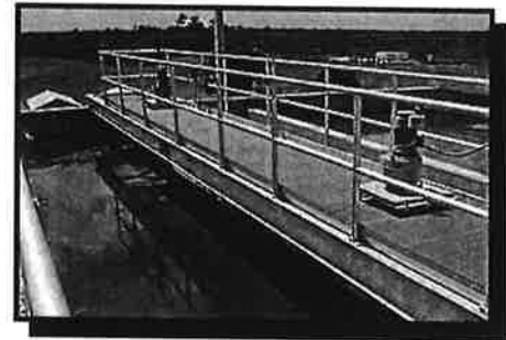
IFAS BNR System: Anaerobic Basins
