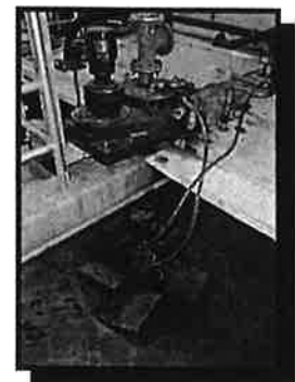
Grit Removal System
