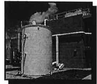
Pretreatment Structure Odor Control System
