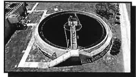
Secondary Clarifier - Conv. ASP System
