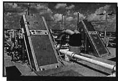
Mechanical Barscreens (3 mm)
