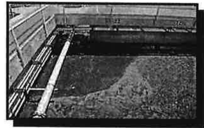
IFAS Secondary Anoxic Basin
