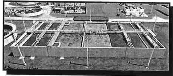
IFAS BNR Treatment System
