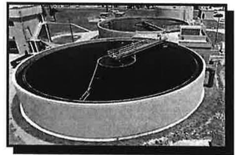
Secondary Clarifiers - Ox. Ditch System
