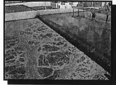
Aerobic IFAS Basin
