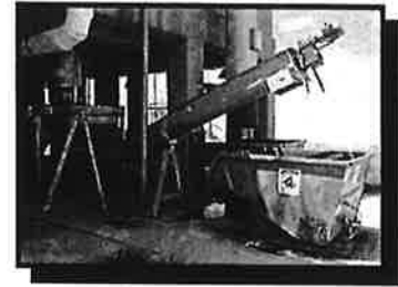
Grit Washing/Dewatering Unit
