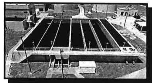
Secondary Effluent CCC/Equalization Tank
