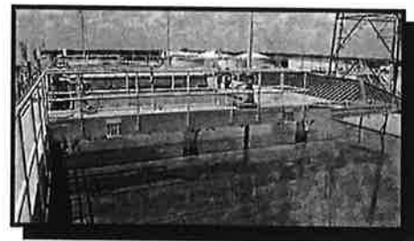
IFAS BNR System: Primary Anoxic Basins
