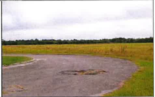
Edisto Road – Deferred Maintenance Near Lot 7
