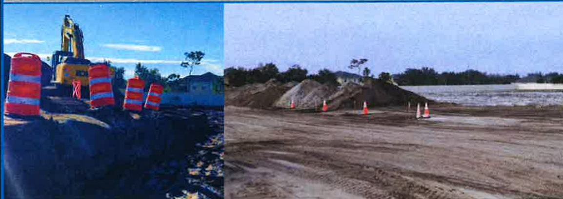
Melbourne Maintenance Facility – Built 1958 Reconstruction of HE Fleet and Central Fleet Underway
