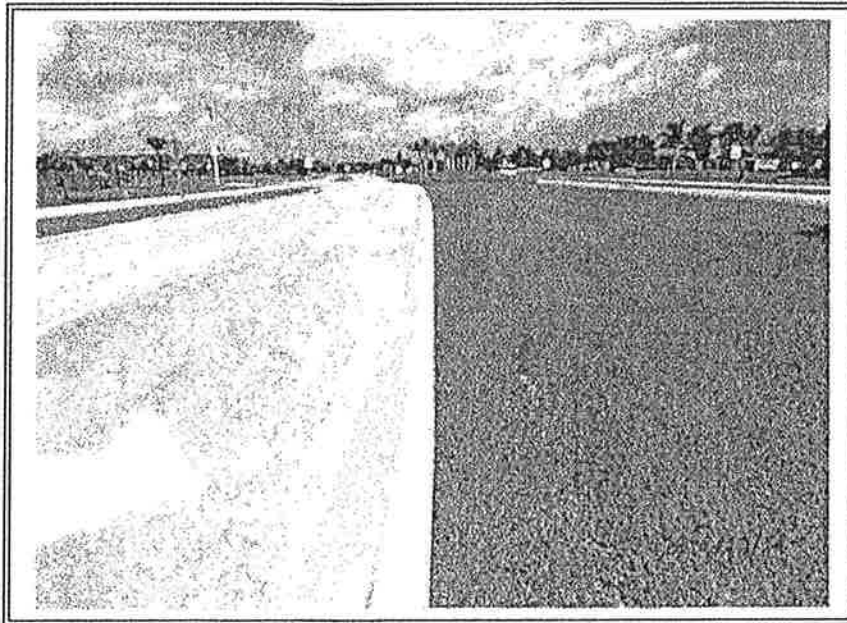
West side of median not consistently sloped at 3 percent to curb
