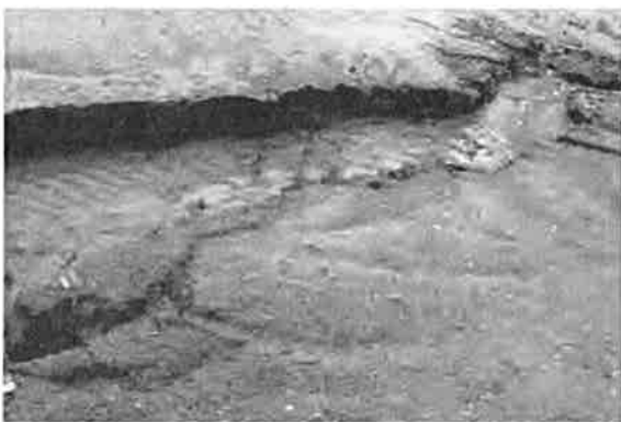
STORM BASIN FLOODING
