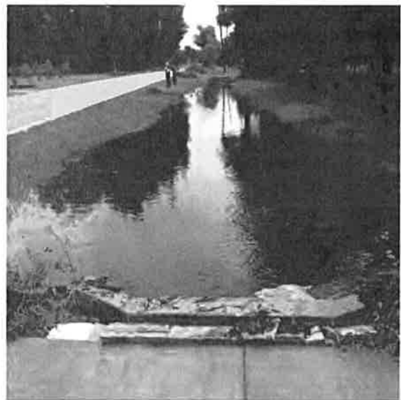
RAIN EVENT EAST SIDE OF ROAD
