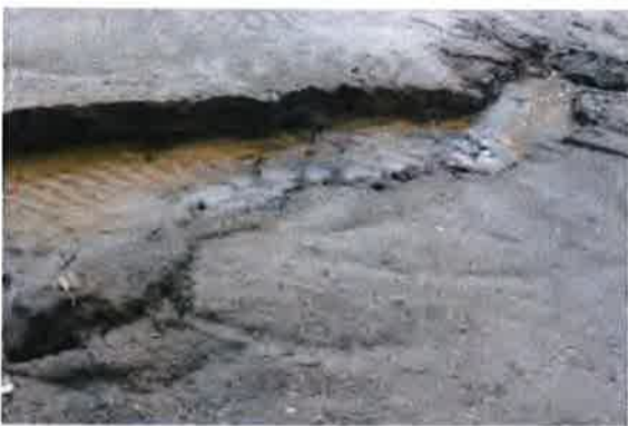
STORM BASIN FLOODING
