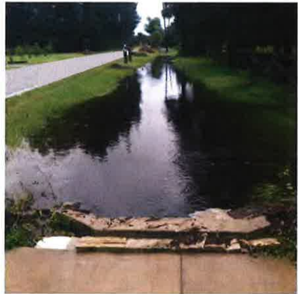
RAIN EVENT EAST SIDE OF ROAD
