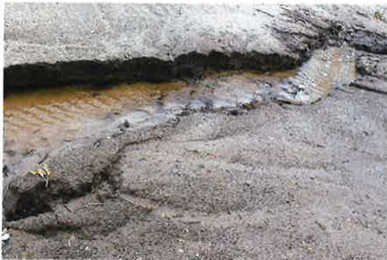
STORM BASIN FLOODING
