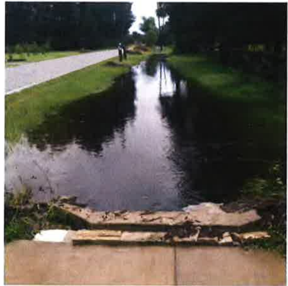
RAIN EVENT EAST SIDE OF ROAD
