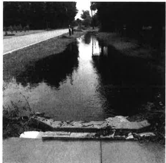
RAIN EVENT EAST SIDE OF ROAD
