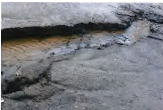
STORM BASIN FLOODING
