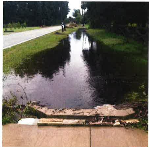
RAIN EVENT EAST SIDE OF ROAD
