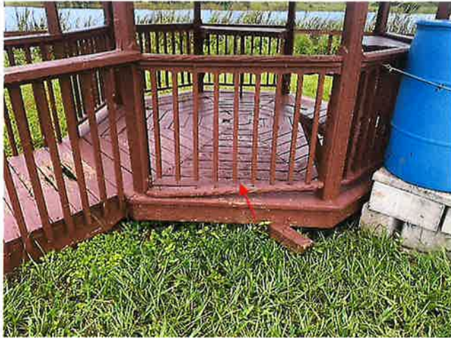
Picture 5 Damaged railing.
