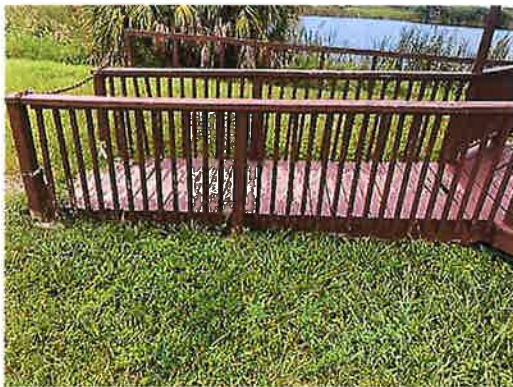
Picture 6 Damaged walkway railing and walkway beam in bad condition.
